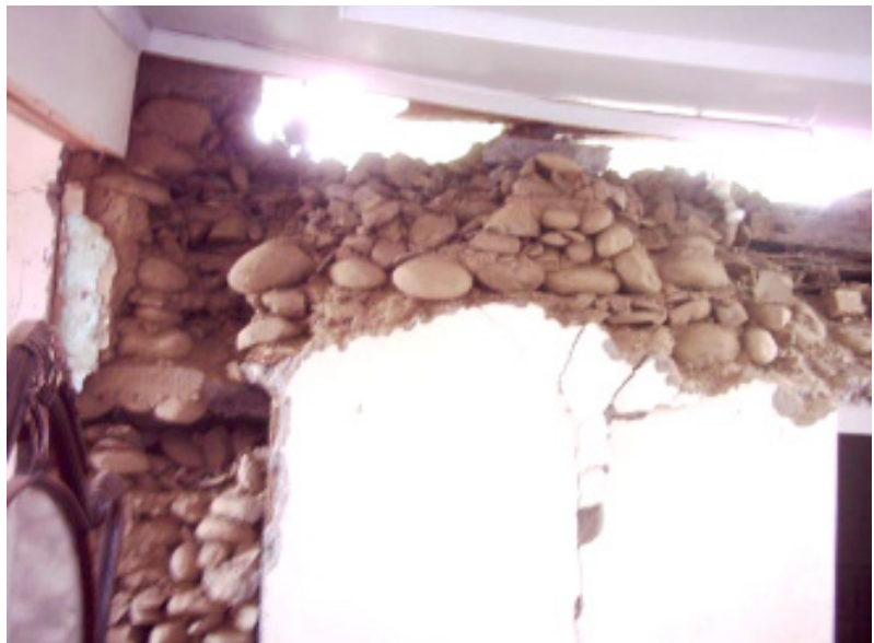
Slika 6. Poškodbe objektov, zgrajenih iz neobdelanega kamna, predvsem prodnikov, s slabo malto Figure 6. Damaged buildings made of unreinforced stone masonry walls
