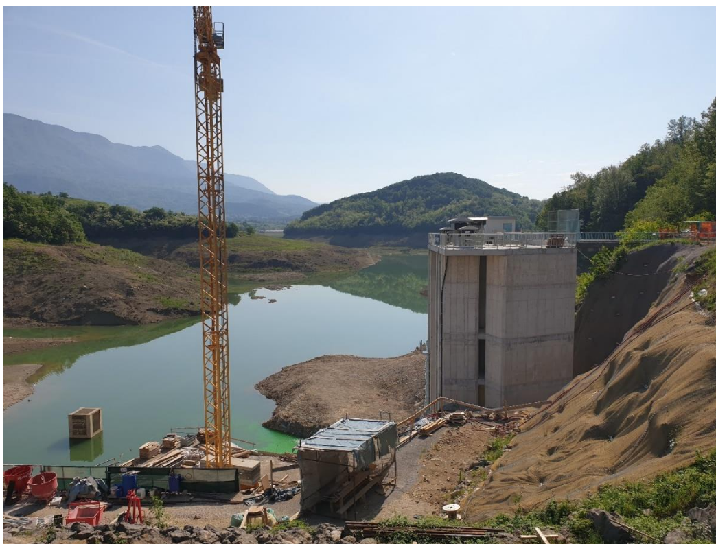
Slika 1. Obnova pregrade vodnega zadrževalnika Vogršček, ki je bil pred tridesetimi leti zgrajen za namakanje polj in nasadov v Vipavski dolini (foto: M. Andjelov) Figure 1. Renovation of the Vogršček water reservoir, which was built thirty years ago for irrigating fields and plantations in the Vipava Valley (photo: M. Andjelov)
