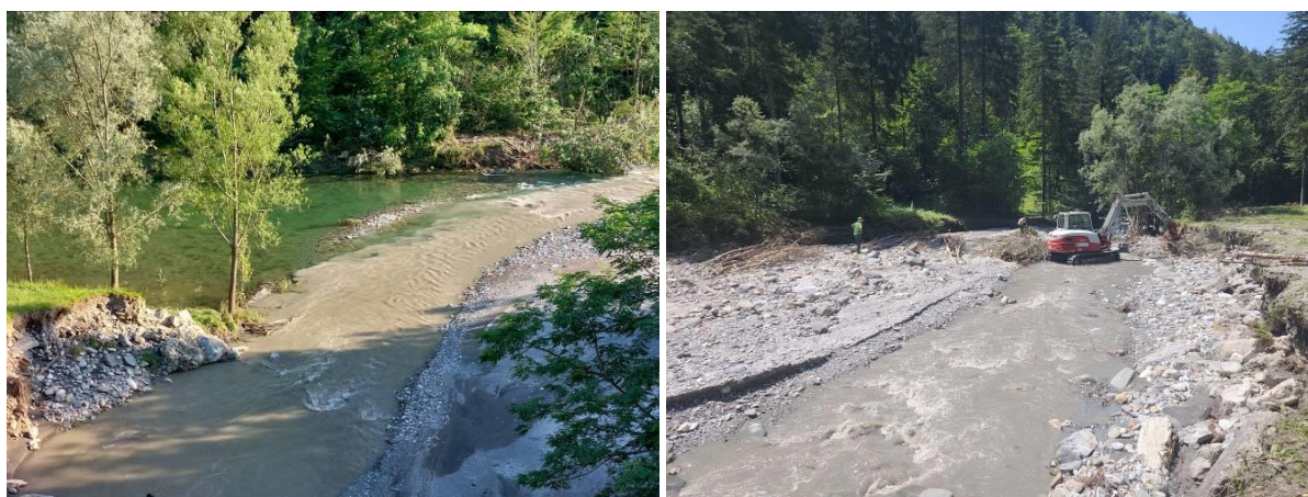
Slika 6. Sanacijska dela po ujmi na Cerknici in pogled na sotočje Cerknice in Idrijce, julij 2023 Figure 6. Remedial works after the flood on Cerknica and a view of the confluence of Cerknica and Idrijca, July 2023
